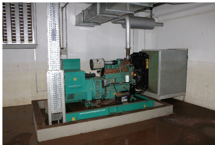
Flooded generator in an airport parking garage
